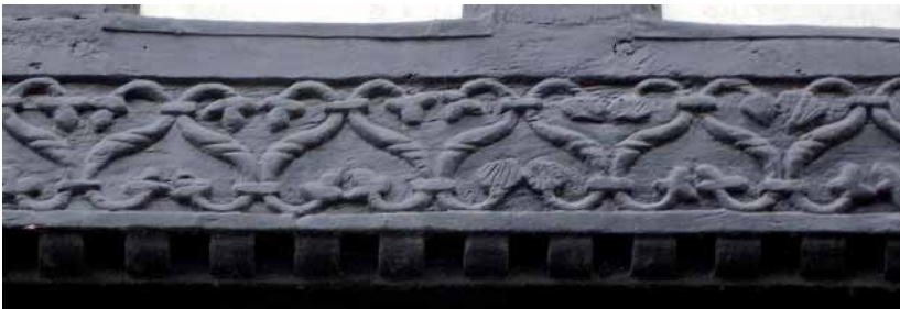
Plate 7. Ornately carved bressumer jetty from a building in Watergate, Chester (Photograph: G.H. Nash)
